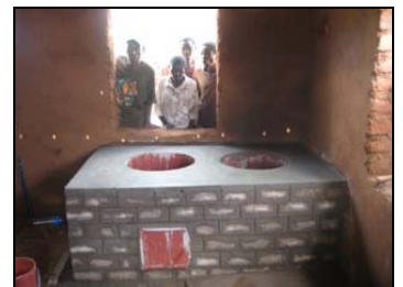
The new stove is ready and can be used after 7 days of curing
