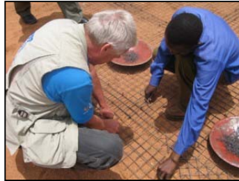
Assisting the construction workers with the iron mesh at Sagara Primary School
