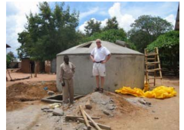
The tank is ready and waiting for pipes and the school building waiting for guttering
